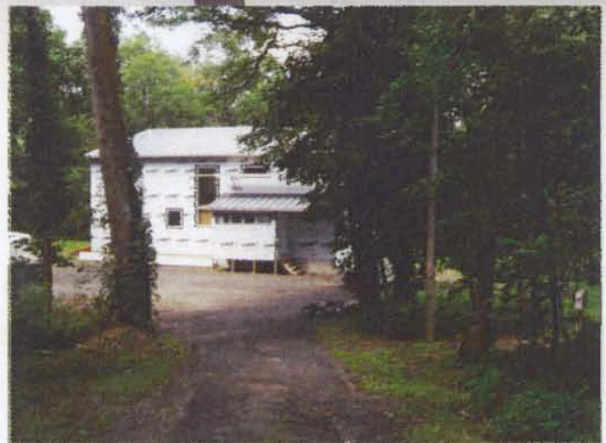
Home Drafty Home. The client's house, built almost 30 years ago, sits on the banks of the Hudson River in New York. It was becoming increasingly difficult to heat in the winter.
