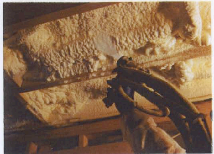
Although the client wanted all applied foam to be closed-cell, Braswell's analysis showed a combination of open and closed would work best for the home's energy efficiency. The crew sprayed 10 inches (25.4 cm) of the open-cell foam on the ceiling.
